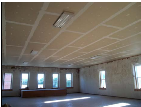
Dance Hall on the upper floor of the Corner Store is ready for renovation. We have plans for a stairway, new door on the west, HVAC and ceiling preparations for painting.
