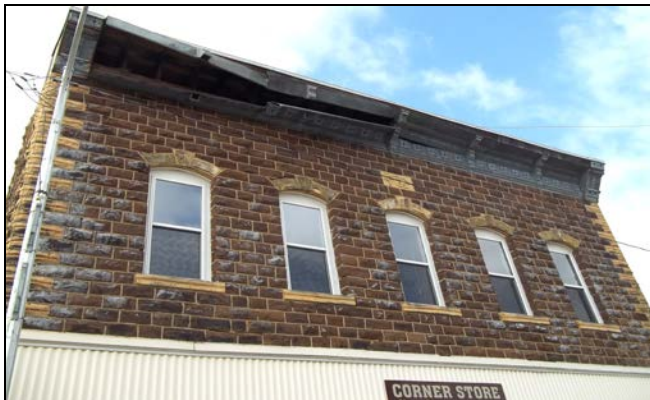
Wind damage from the June 27 th storm.
